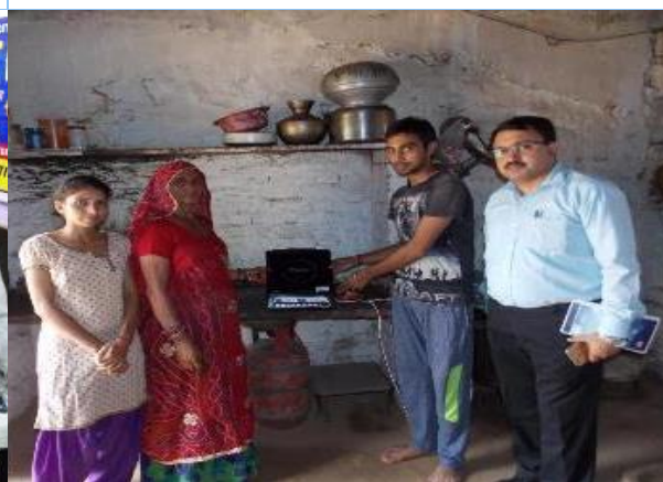
Installation of induction cooktops in kitchen and checking the wiring and plug points – Ensuring quality
