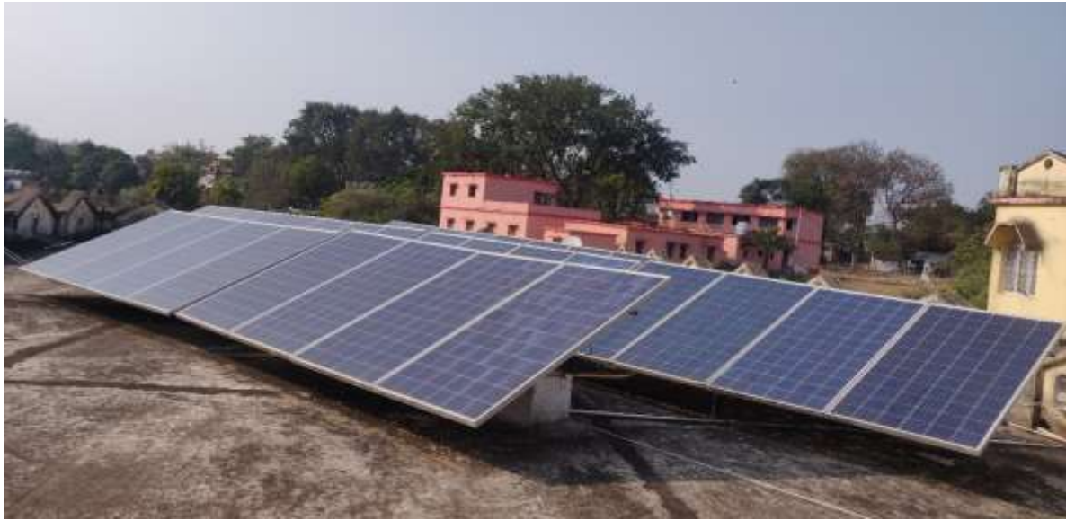
Figure 1 Rooftop solar panels at a residential school in Ranchi
