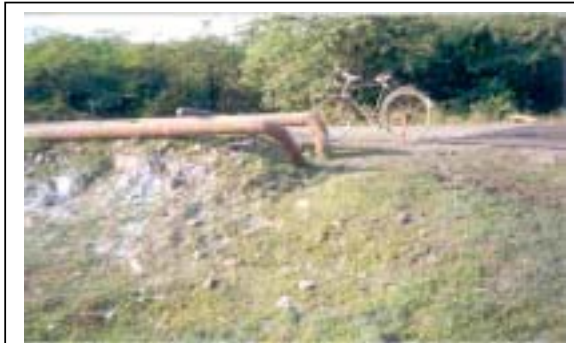
Photo 4.2: Ash disposal pipe from boiler to ash pond.
