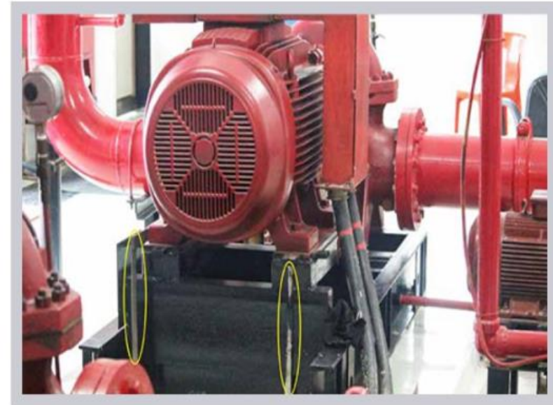
Motor double earthing
